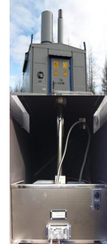
Thermoelectric stations for gas pipe lines http://www.telgen.ru/
